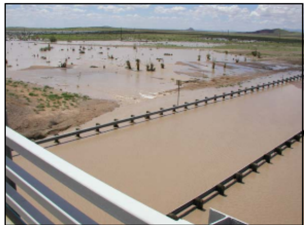
Figure 11: Interstate 10 between Las Cruces and Deming on August 28, 2006, closed due to flooding. Photo by Bruce Bradley/NWS.
